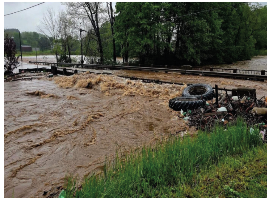
On May 14, 2025, torrential rains swelled Piney Creek, a tributary to the Casselman River, and caused extensive damage to the 102-year-old bridge in the village of Boynton.
