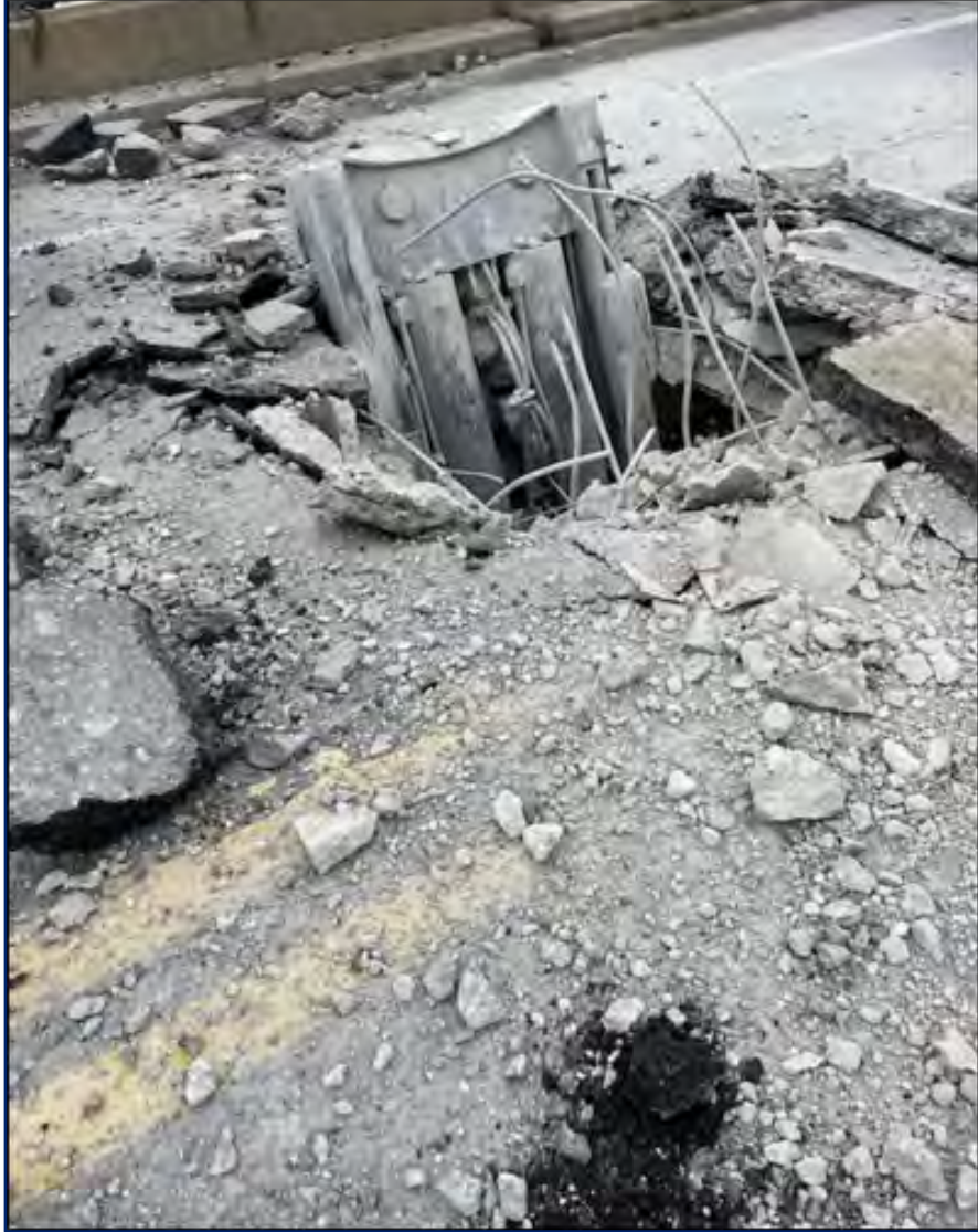
Damage to bridge deck
